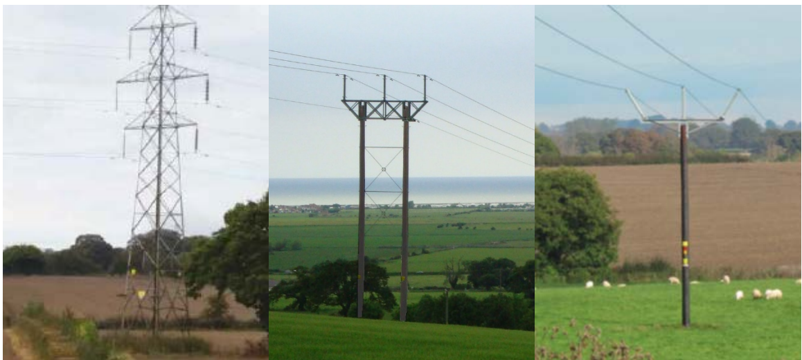
Steel pylons – approx. 26m
